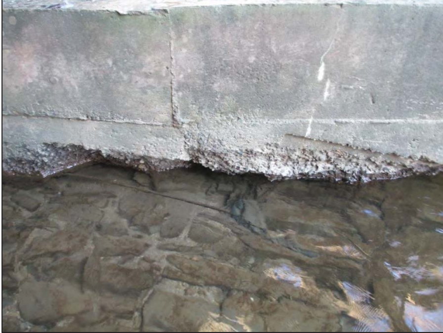
21: Close-Up View of the Far (North) Abutment Apron at the Upstream Corner Note – The concrete apron exhibits moderate to heavy abrasion along the waterline with several pockets of undermining measuring up to 1' D lateral penetration.
