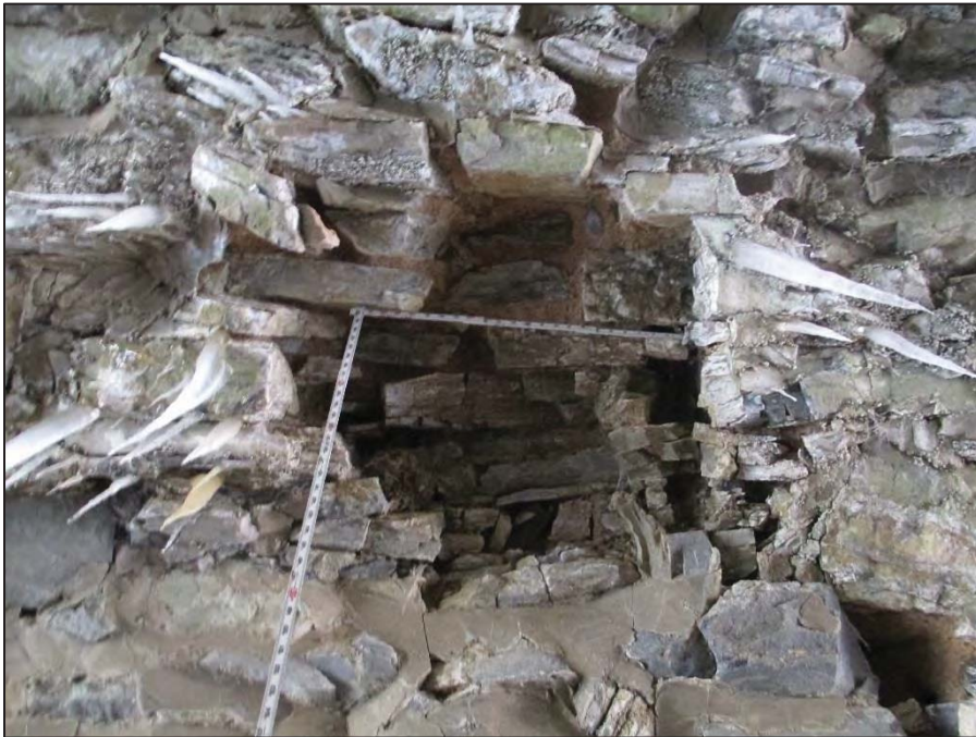
10: Close-Up View of the Superstructure Underside
