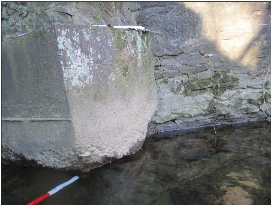
22: Close-Up View of the Far (North) Abutment Apron at the Upstream Corner Note – The apron is undermined 3' D x 2' H at the upstream corner.
