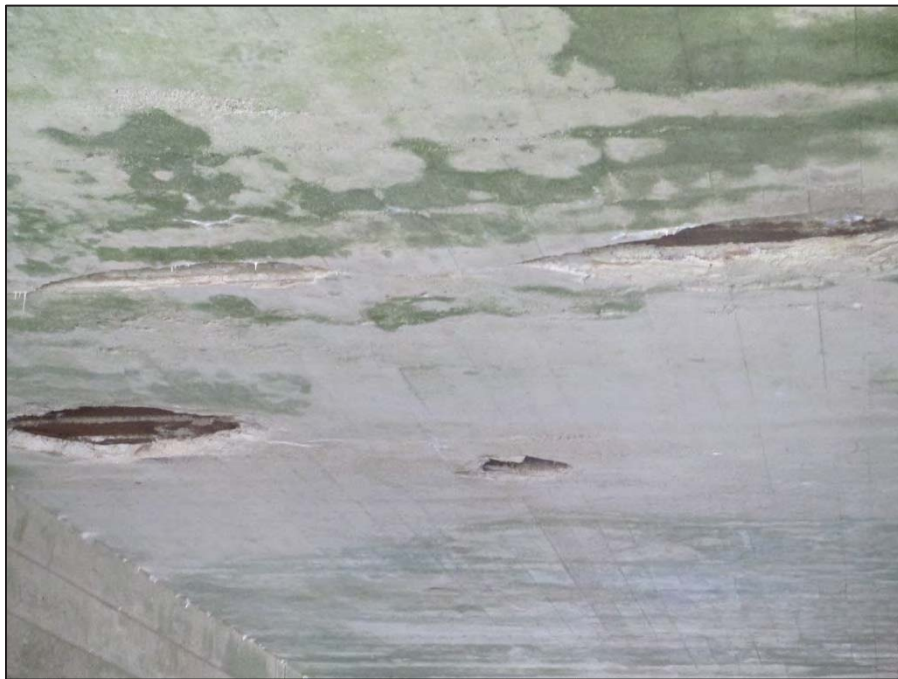
10: Close-Up View of the Superstructure Underside Note – There several spalls with exposed I-beam bottom flanges near mid-span.
