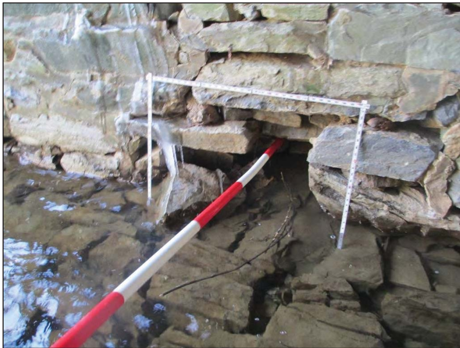
16: Close-Up View of the Near (South) Abutment at the Upstream Corner Note – There is a 2' W x 2' H x 1' D area of stone and mortar loss.
