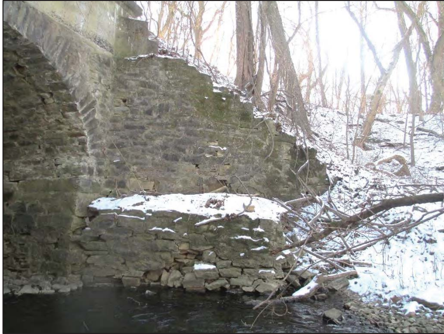
17: General View of the Near Left (Southwest) Wingwall Note – The buttress wall exhibits numerous areas of missing stone and mortar.
