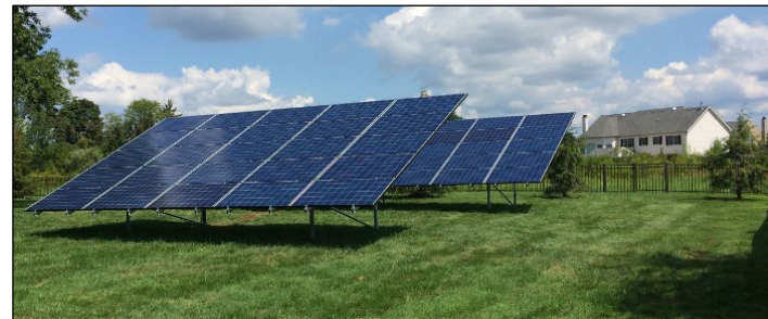
Source: Exact Solar
