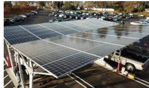
Source: Exact Solar
