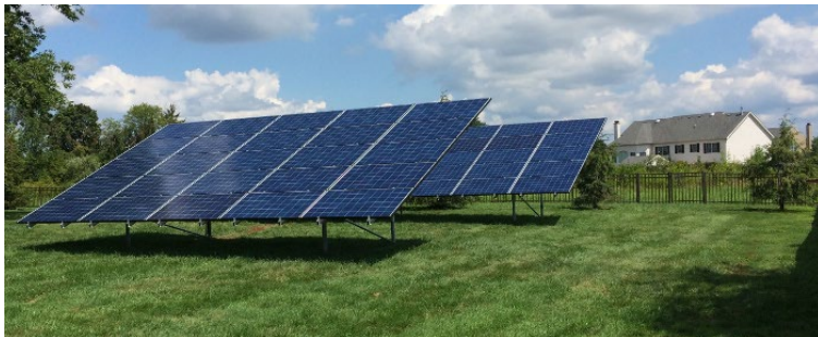
Source: Exact Solar
